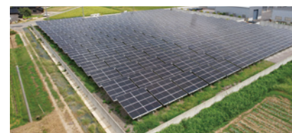
Ground mounted solar power plant for off-site PPAs
