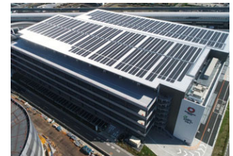
Onsite PPA installed on rooftops
